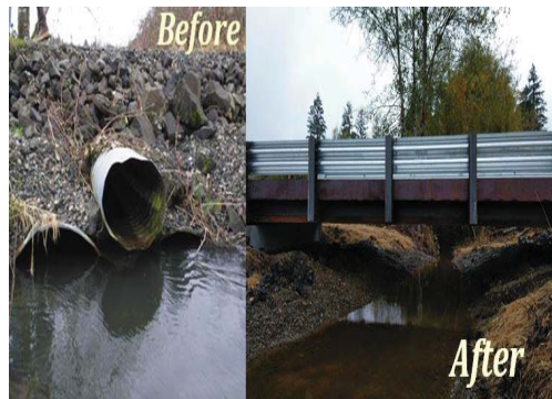
A clear before and after of the blockage, and resulting open flow of the creek. Photo by Nora White
