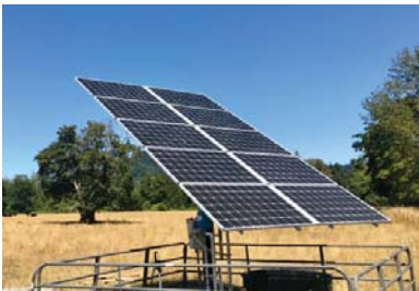
Thurston CD helps local farms convert to renewable energy! This solar pump was installed on a South Thurston cattle ranch! Photo by Kevin Jensen, Riverbend Ranch
